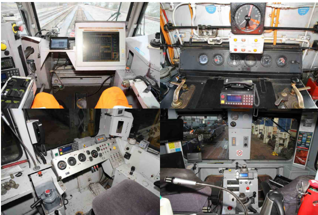
Will ERTMS screens fit into the already cramped cabs of many on-track machines? João Gaspar presentation.
