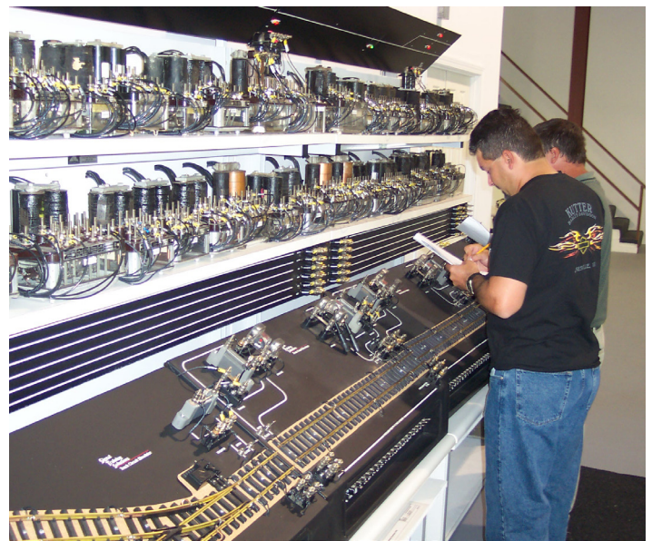
Training on relay use in the United States. Photo Big J Railway Signal Enterprises.
